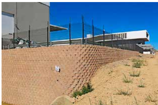
Terraforce retaining blocks lining a slope bordering a detention pond.
